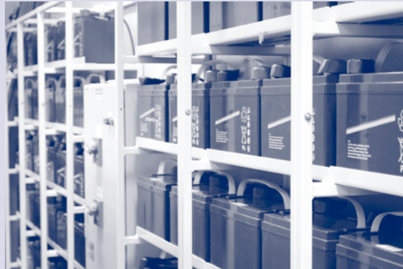
Banks of Batteries
