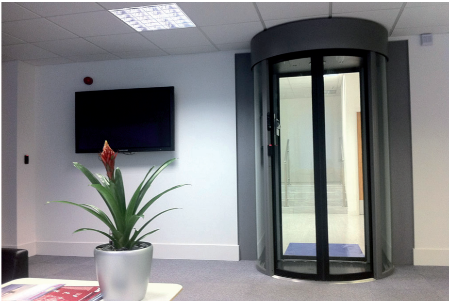
FIGURE 19.2 A mantrap installed in a lobby
